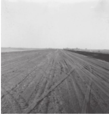
1. A new style drain, 5 miles south of Smith Siding in 4-1W. The spoil bank has been smoothed out into a wide road bed, and the sides of the ditch have gentle slopes. No seeding as yet.
