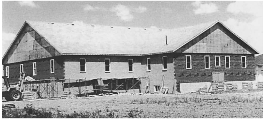
Construction of the new Kingsville Old Colony Mennonite Church, 1997. Photo by George Schartner and courtesy of Biographies of our late Leaders, page 31.
