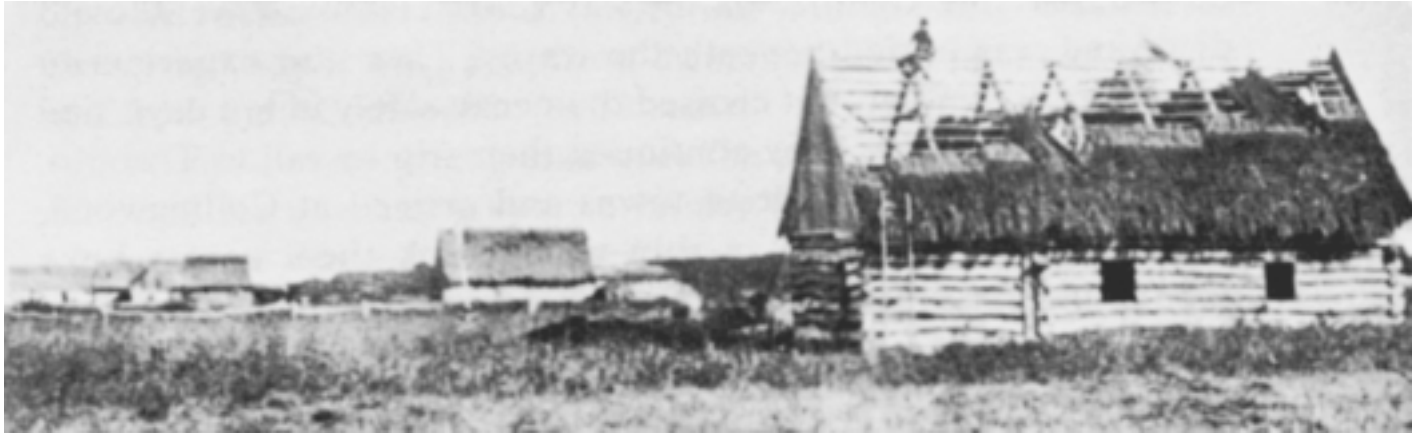
Building the first Old Kolony school in the village of Blumenort on the West Reserve. The village was one of the very first to be built in that area in 1875. Photo and caption courtesy of Man. Men. Memories 1874-1974 (Altona, 1974), page 26.
